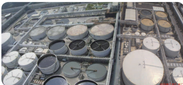
Wastewater treatment plant (Before improvement)
